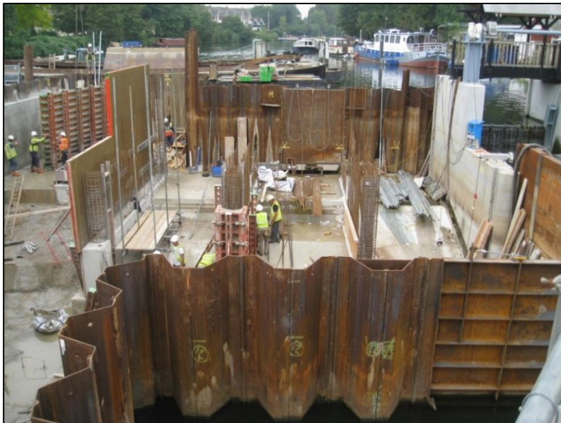
Plate 4-6 - An example of a coffer dam, used to construct new weir gates.
