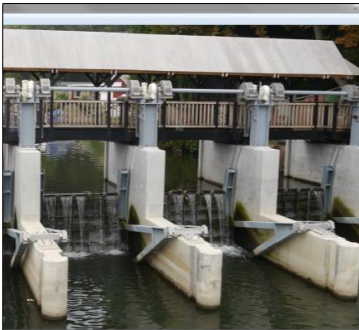
Plate 4-4 - An example of an existing River Thames radial gate weir at Molesey.
